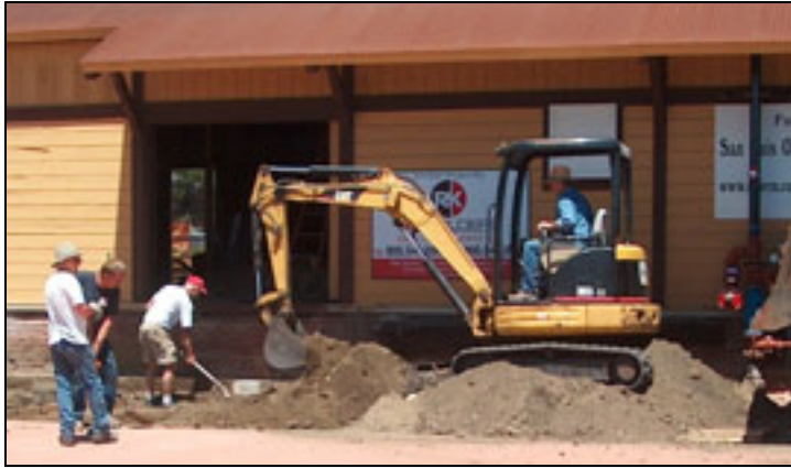
Museum volunteers Chris Hurd, Ted VanKlaveren, Robert Evenson and Alvin Evenson labor to prepare the site for the Pacific Coast Railways boxcar #706 to be installed next to the Freighthouse. Photo by Glen Matteson
